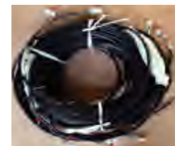
CALLING ELEVATOR CABLE
